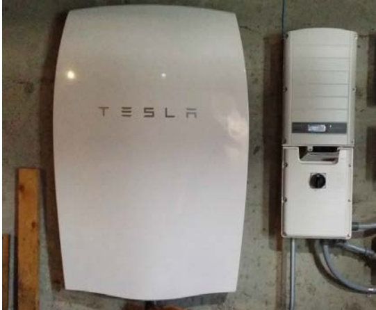
(a) Tesla Powerwall
