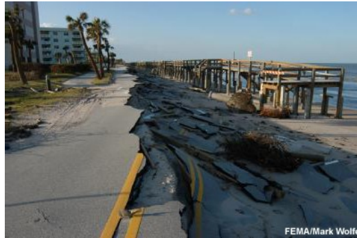
(a) Beachfront Road and Boardwalk Damaged by Hurricane Jeanne (2004)
